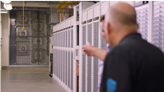
Figure 9- Fan wall inside Microsoft's fifth-generation data center in Quincy, Washington (Source: Microsoft video) 9
