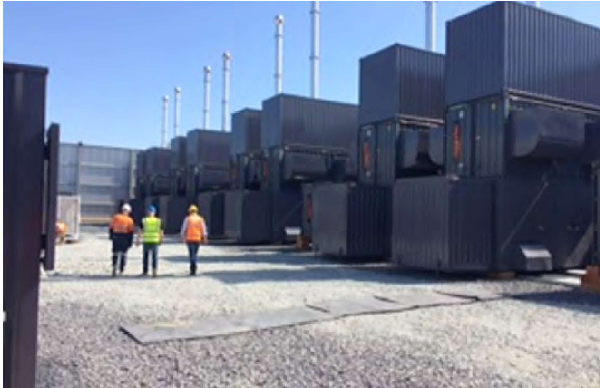
Gas generators powering data centre - up close.
