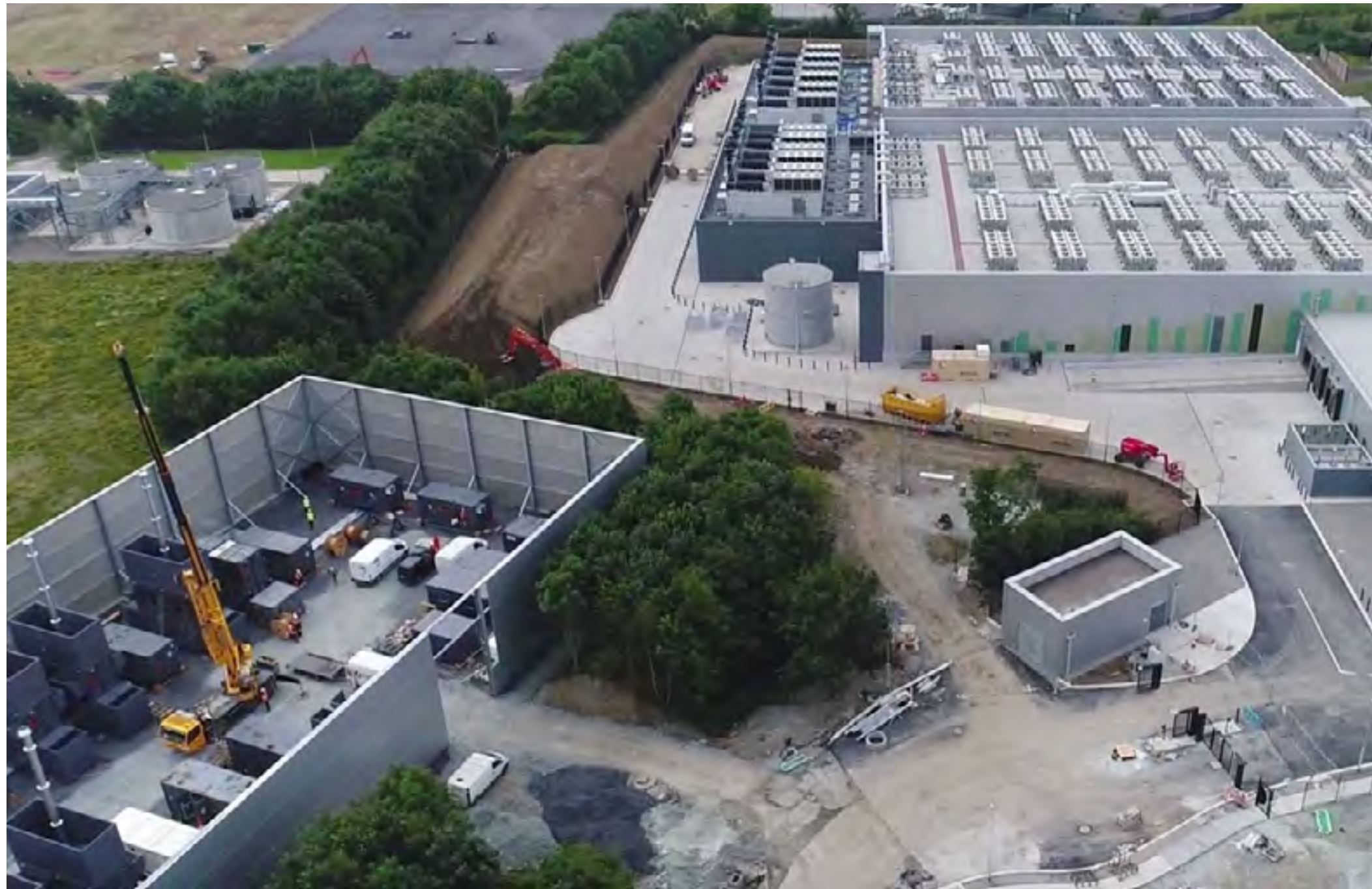
Gas generation compound in construction at data centre in Ireland.
