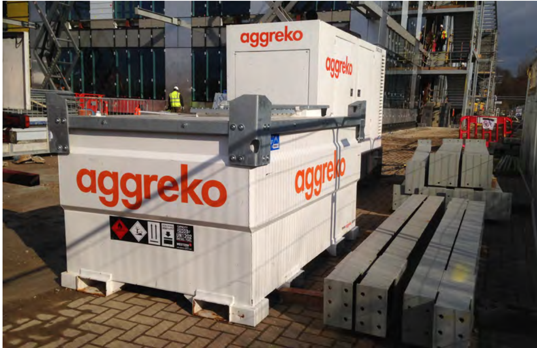
Canopy generator and fuel tank at data centre construction site.
