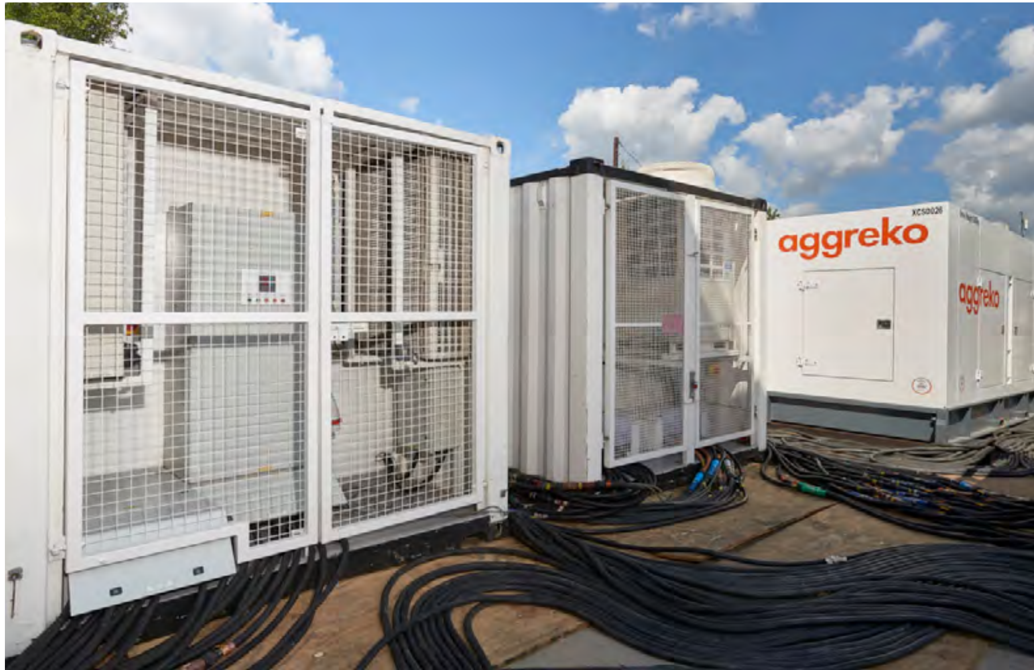
2 x 500 kVA UPS system for a data centre in Ireland following a Saturday morning call for emergency power.
